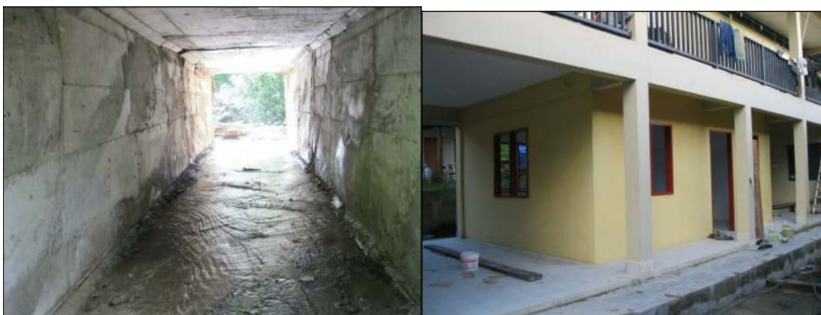
(left) view of the BRS access road box culvert (25 February), showing poor quality of workmanship, (right) new BORA office (24 February), located on the ground floor of Rumah Badak.
