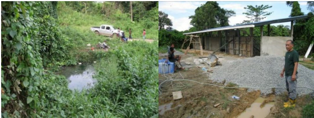
(left) a spring (“mata air”) exists within 80 metres of the Rhino Quarantine Facility, but it was found to dry out during non-rainy periods, and being near the public roadside there is a risk of pollution, so is unsuitable as a water source, (right) construction of the RQF underway in late June.
