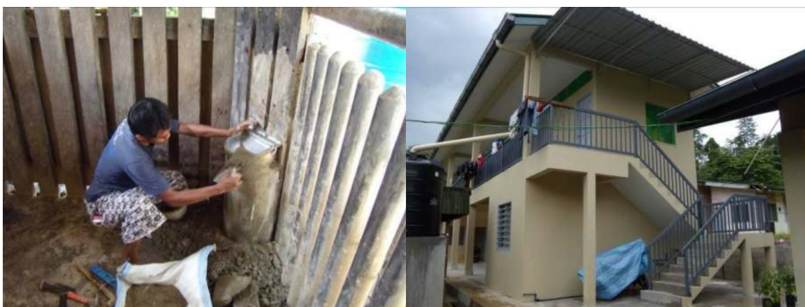
(Left) Installation of drinking water dispenser in the night stalls, to minimize both wastage and fouling of rhino drinking water. (Right) Completed Rumah Maitap accommodation for BORA field staff.
