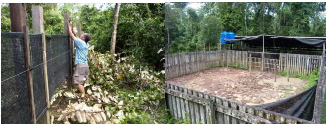
(Left) Repair to the interim rhino paddock fence, damaged by a branch fall. (Right) A temporary breeding paddock (optimistically assuming Tam and Puntung may get together before the permanent BRS construction) was made in July by modifying two old (1990s)
