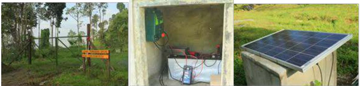
Rhino food garden development at Tabin at end of March 2013, (left) entrance to the 2 hectare garden, (middle) energizer battery which powers the electrical wires of the perimeter fence (to prevent elephants from entering the garden), (right) the solar panel which powers the energizer
