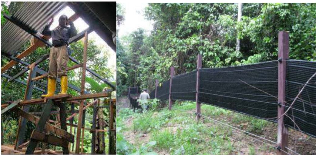
(left) construction of extra staff quarters space at Rhino Interim Facility (October), (right) completed additional rhino paddock at Rhino Quarantine Facility (RQF; November)
