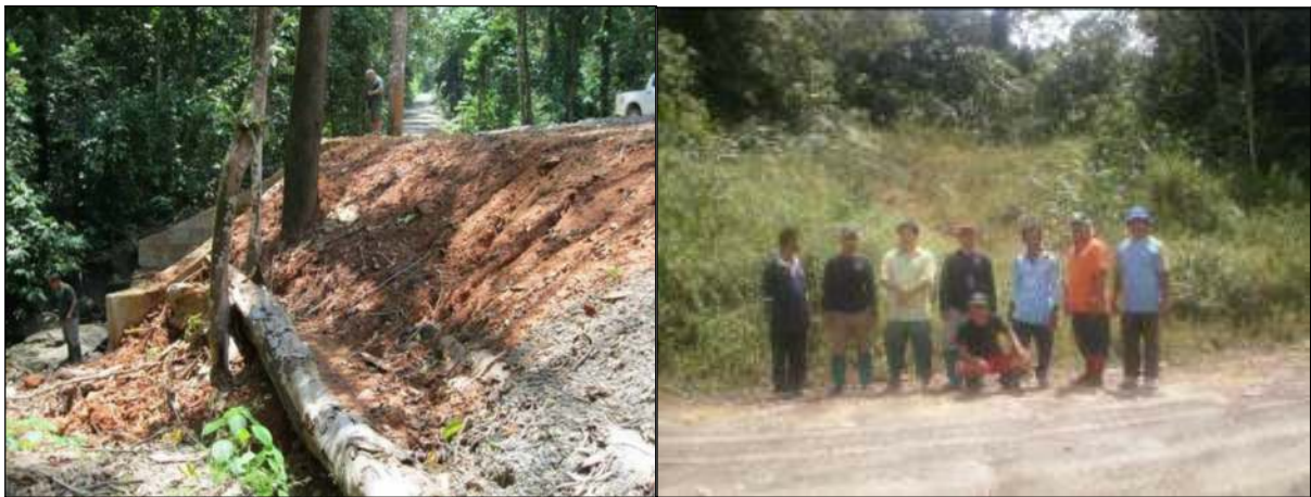
(left) BRS access road, early August, showing bare soil embankments near culvert, (right) Tagason area in upper Kuamut region, where rhino footprints were seen by people from Kampung Kuamut in 2009 (photo : Rasaman Jaya)
