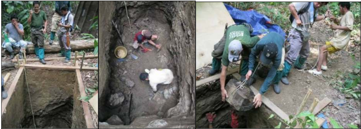
(left) digging the hole for trap 5, (middle) a view inside trap 5 hole during construction, the rock is removed by chisel and pick axe down to a depth of eight feet, (right) removal of rocks from the trap 5 hole during construction.
