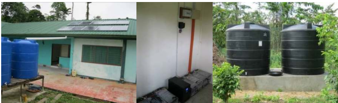
(left) the ten photovoltaic cells for solar electricity at RQF were installed in mid November, (middle) the electrical storage batteries, (right) the piped water supply to RQF remained unconnected by end of this quarter, and the two new water storage tanks at the RQF had to be filled manually.
